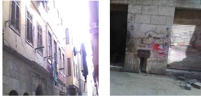
Fig (6) shows a few of deterioration after rehabilitation according to absence of maintenance
